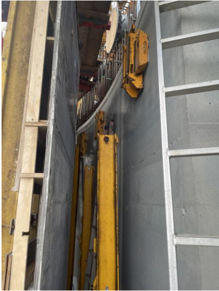
Figure 11: As a preparatory step for platform climbing, the ACS needs to raise the climbing rails to form the track. Although the structure is relatively vertical between Levels 104m(U30) and 184m (U49), it becomes narrower as the height increases. Therefore, the climbing rails of each platform must incline not only forwards and backwards but also left and right during climbing. By switching the remote control, hydraulic control for each unit is possible, allowing for fine adjustments.
