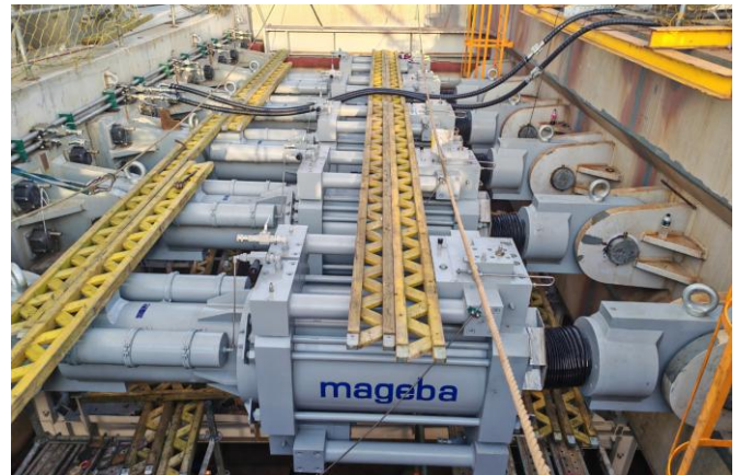
Figure 11: HFR array installed and interlinked
