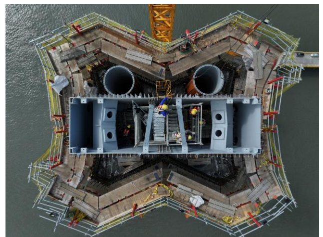
Figure 10: The self-climbing system eliminates the risk of falling by ensuring that all eight platforms climb simultaneously. On the other hand, the pump control allows each unit (with two cylinders) to operate the cylinders independently. This means that in case of any issues, we can respond quickly and flexibly with just a single button on the remote control
