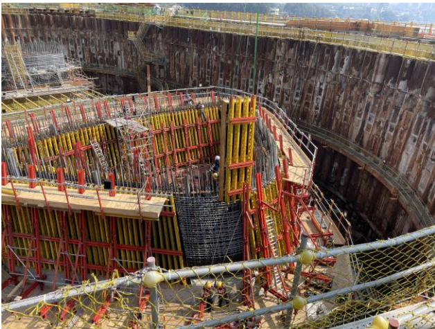
Figure 3: Wall Formwork VARIO+3D Boxes adapt 3D curve geometry. The optimised 3D box sections were reused to plan cost-effectively
