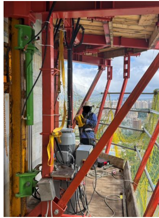
↑ Figure 40: Hydraulic cylinders and pump on level -1 – heart of ACS. The operator controls the climbing of all ACS units with a single push of the remote control button
