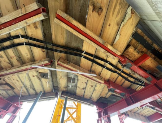
Figure 39: Telescopic cantilevers on ACS Level 0
