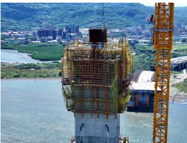
Figure 9: ACS self-climbing system. After completing concreting at Level 104m (U29), we gradually installed the ACS. The self-climbing successfully covered the range from Level 104m (U30) to Level 184m (U49)
