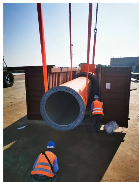
Figures 19 and 20: Lifting of an element and its placing in the container
