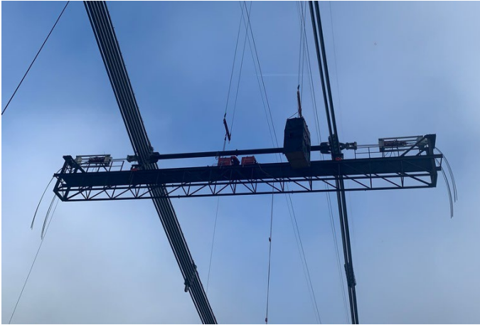
Figure 21: Strand jack widening unit at the time of spread beam installation / schlaich bergemann partner
