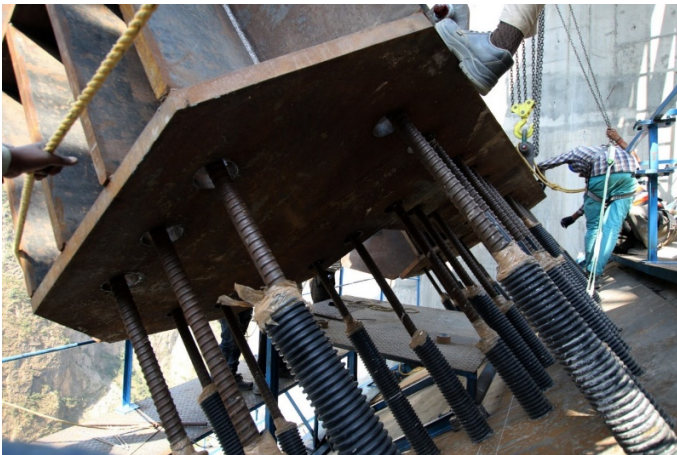
Figure 21: Lowering the base segment in the correct position to match the drilling holes for the pre-installed anchor – heavy work on site around 200 m above the ground and 50-degree inclination
