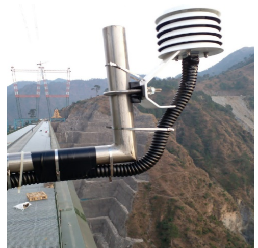
Figure 6: Air temperature sensors
