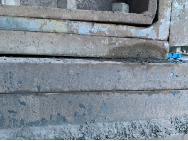
Figure 4: Steel elements that are not evenly supported lead to uneven application of force and pose a problem for corrosion protection
