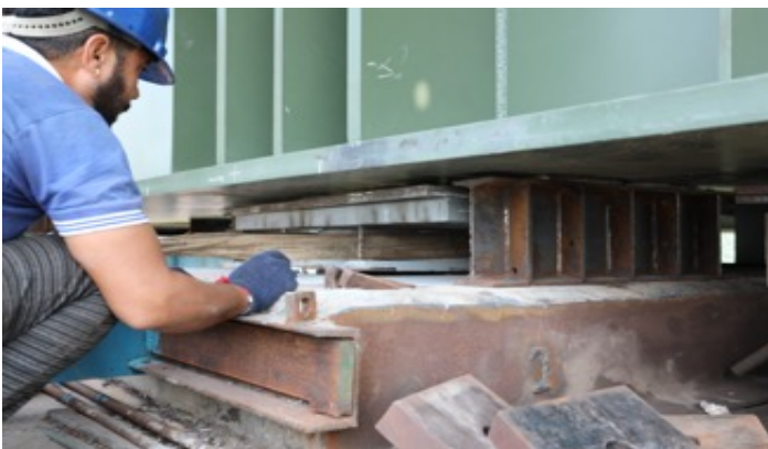
Figure 6: Bearing installation with gap between upper bearing plate and bridge girder
