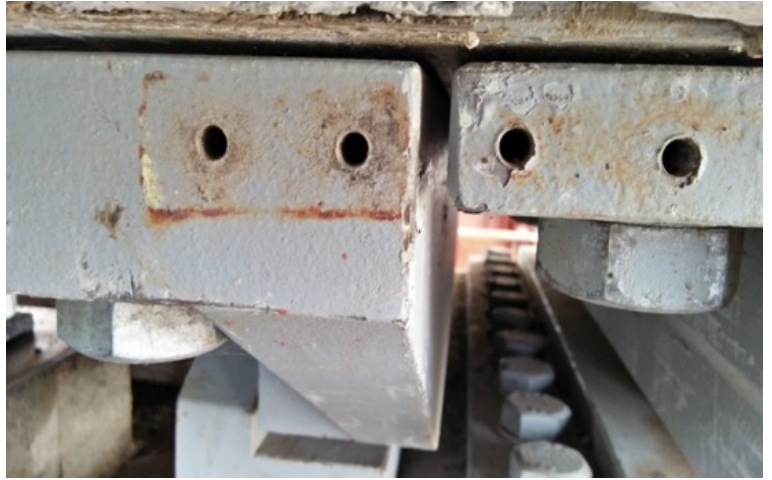
Figure 5: Typical gap situation observed in bearing installation
