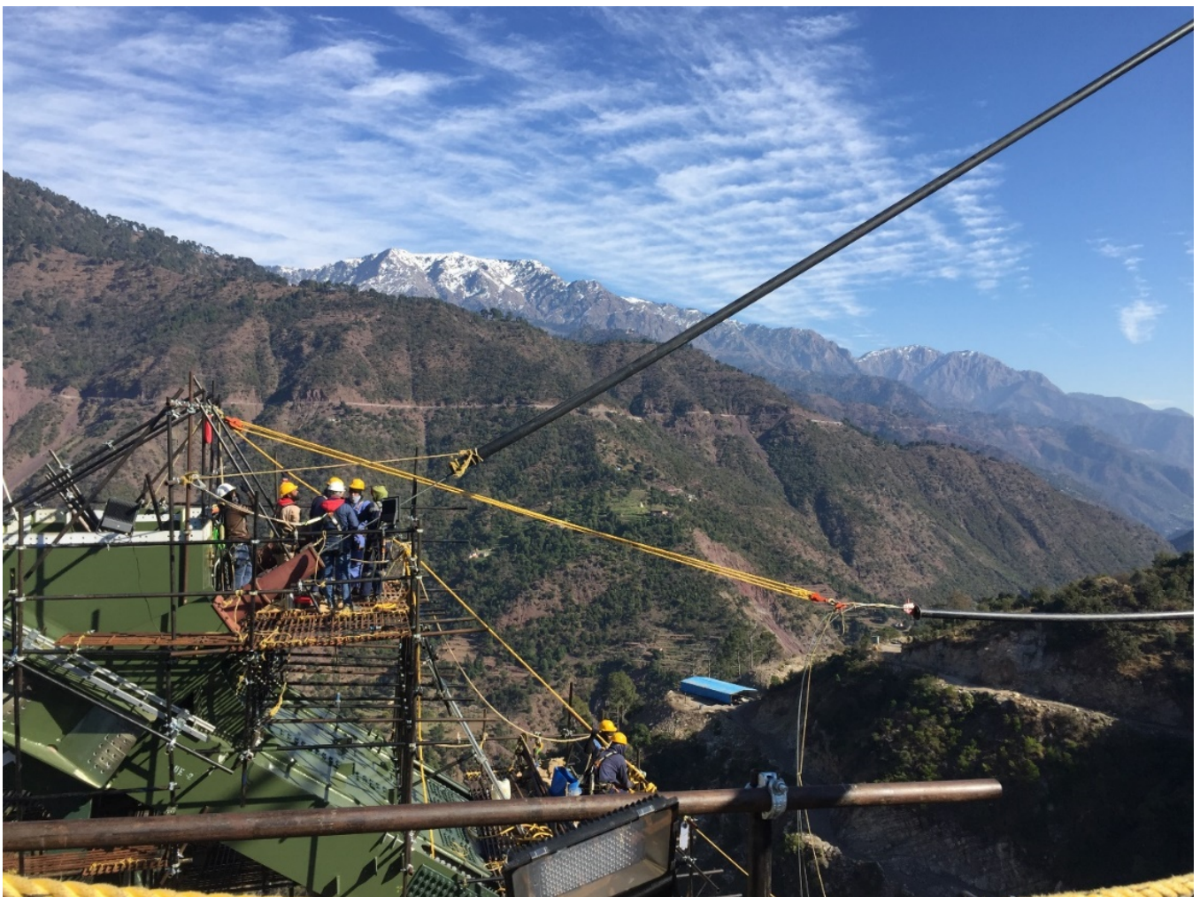
Figure 2: Arch – stay pipe with 1 st strand installed; another stay pipe being installed
