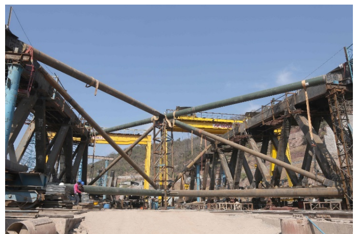
Figure 18: Trial assembly of a part of the arch on ground – installation of 3D wind bracing
