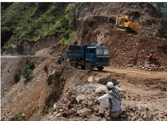
Figure 3: Building new roads in the mountains on the way to site for the Chenab Railway Bridge
