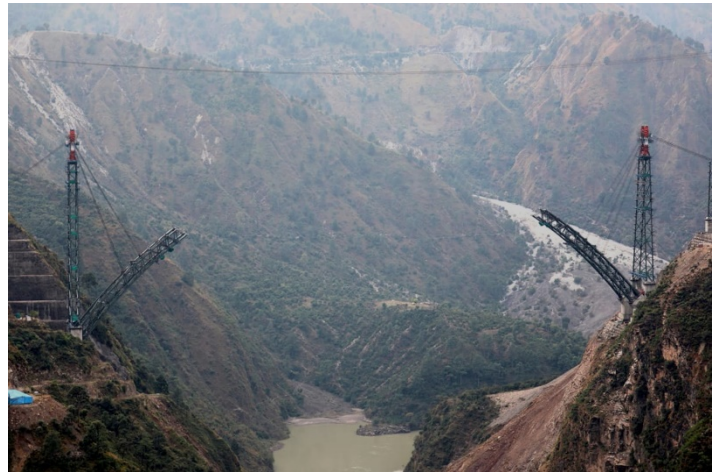
Figure 33: Assembly situation after installation of the second anchorage cable; the assembly process was stable and safe
