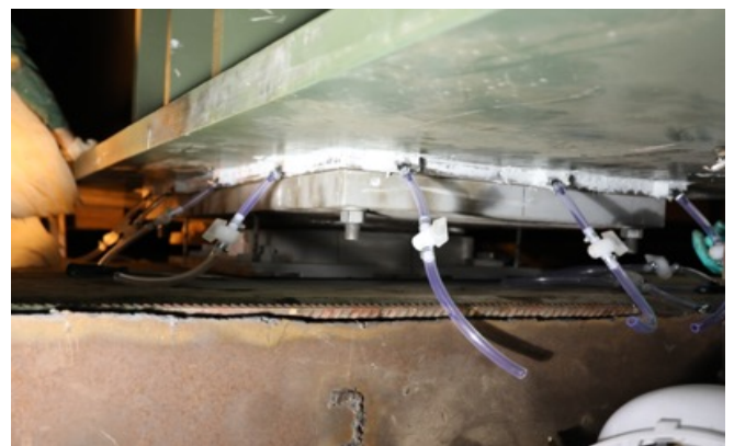
Figure 7: MM1018 application between upper bearing plate and bridge girder to ensure 100% connection of the bearing to the bridge
