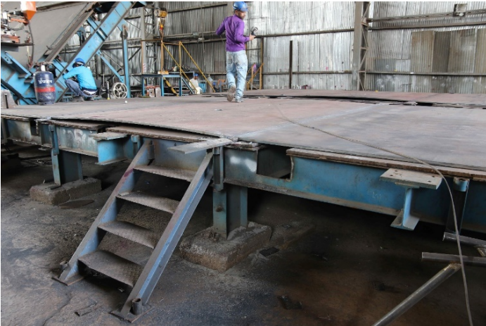
Figure 26: Distortion of web plate – post heating
