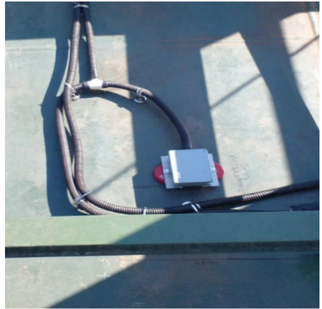
Figure 7: Accelerometer installed on the deck
