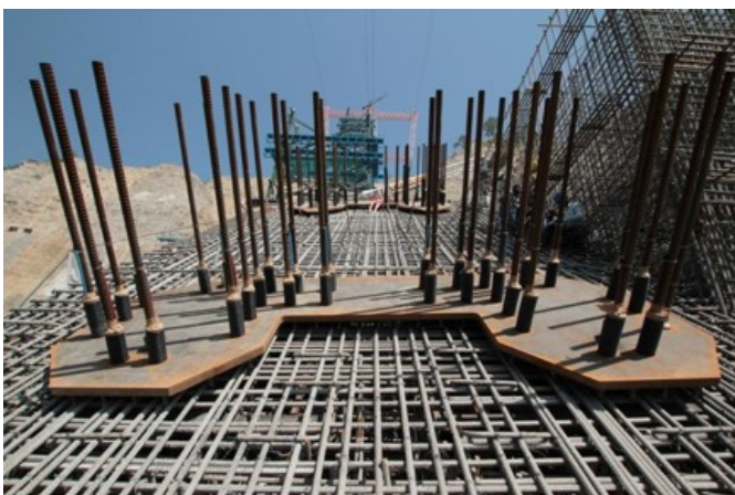
Figure 19: Part of the base plate fixed on reinforcement with pre-installed anchor bars
