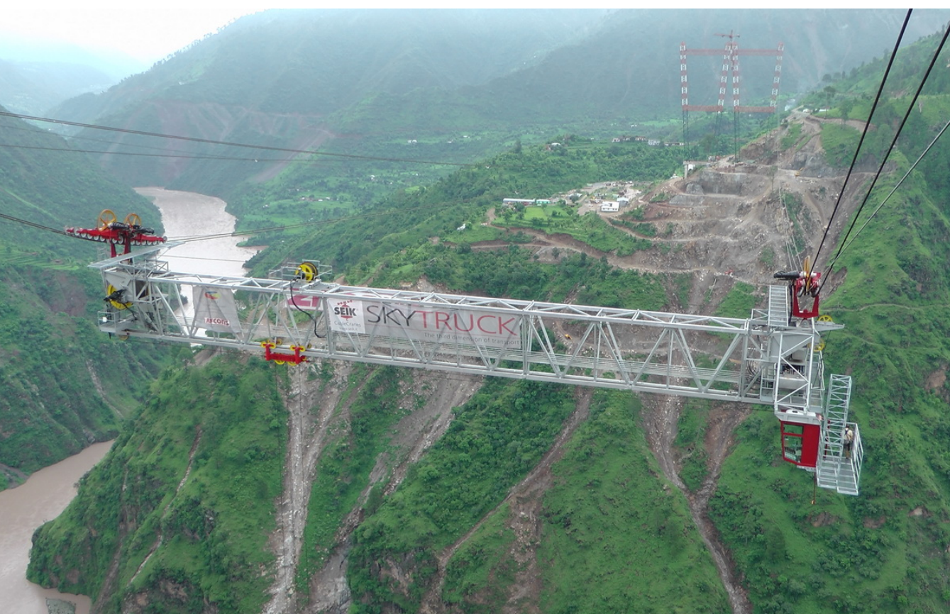
Figure 3: Skytruck 200 ready for operation
