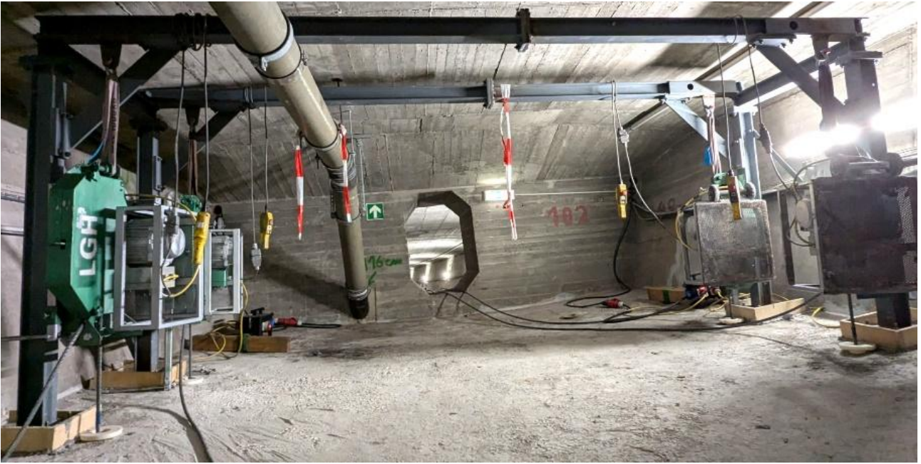
Figure 4: The cables passing down through the box girder on the left and right
