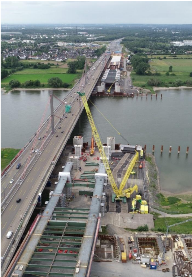
Figure 12: Side span construction with crawler crane Source: Die Autobahn GmbH des Bundes
