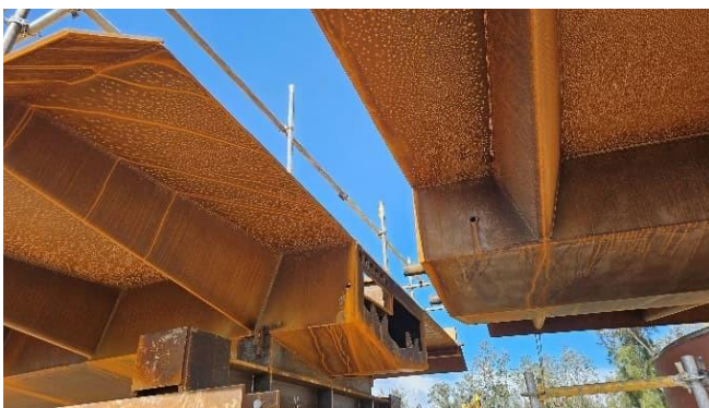
Figure 19: Stabbing guides to efficiently align and join bridge segments with the receiving unit on the left and guides on the right module
