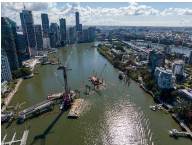
Figure 25: Under construction for almost three years, the Kangaroo Point Bridge has quickly become an important element of vibrant Brisbane CBD. Construction started in January 2022 and was completed late in 2024, with the bridge opening on 15 December 2024
