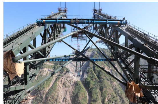
↑ Figures 10b and 10c: Erected 1 st set of wind bracings with access platforms in span S40A-S41 & S50A-S49
