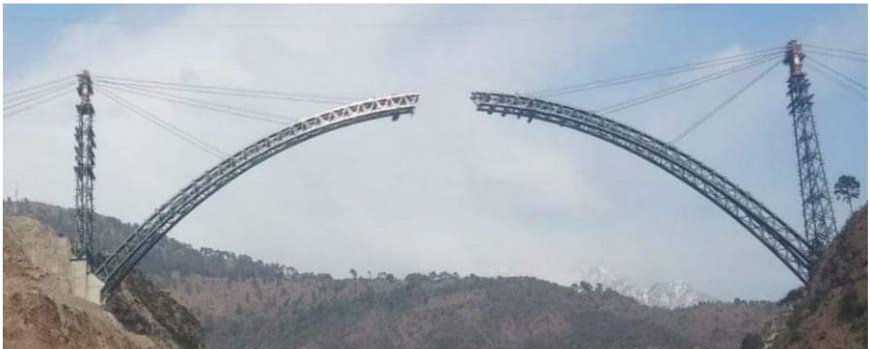
Figure 19: Photo showing arch erection from both sides and last three cables just before arch closure
