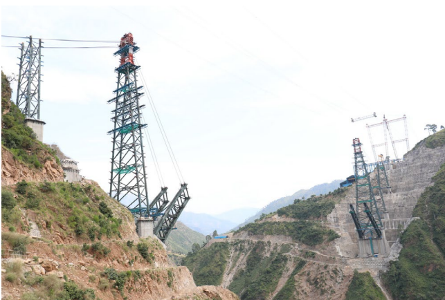
Figure 14: Photo showing erected Arch girders and the first set of stay cables
