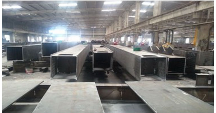
Figure 4a: Typical cross section of the arch and photo of fabricated single boxes in shop
