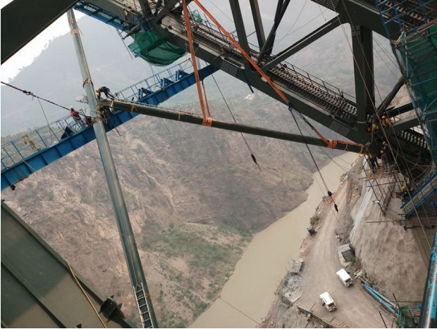
Figure 10a: Erected wind bracing 40m pipe with connecting pipe at bottom chord level
