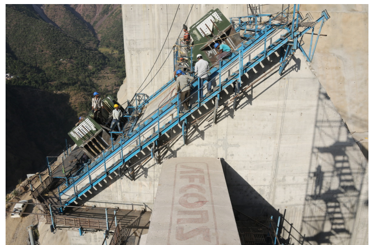
Figure 13: Arch foot layout and installation Click on the image (left) to open it in a higher resolution
