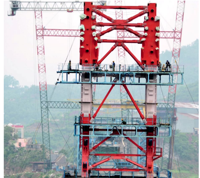
Figure 13: Temporary tower above pier during erection (left) and after erection completed (top)
