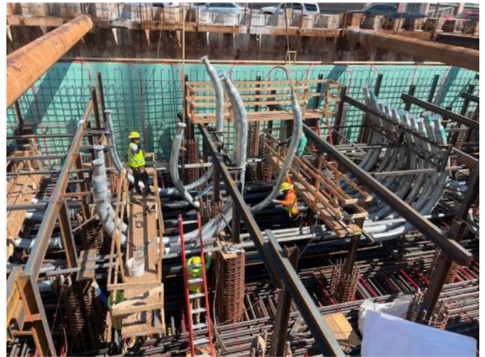
Figure 6: Footing construction. The curved, galvanized steel route post-tensioning cables from the arch ribs to anchorages that are accessible at the top of the footing.
