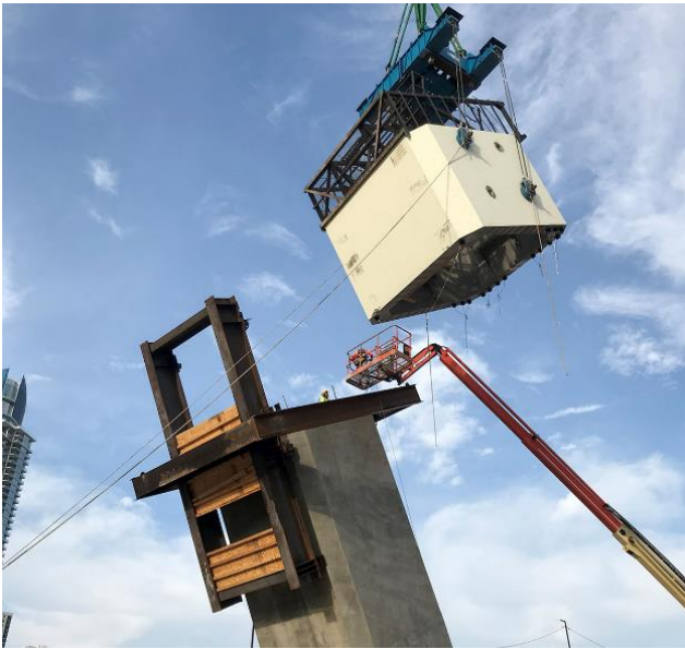
Figure 13: Precast segment being placed at the top of the cast-in-situ arch starter. The starter frame is used to stabilize and adjust the segment prior to casting a wet-joint.
