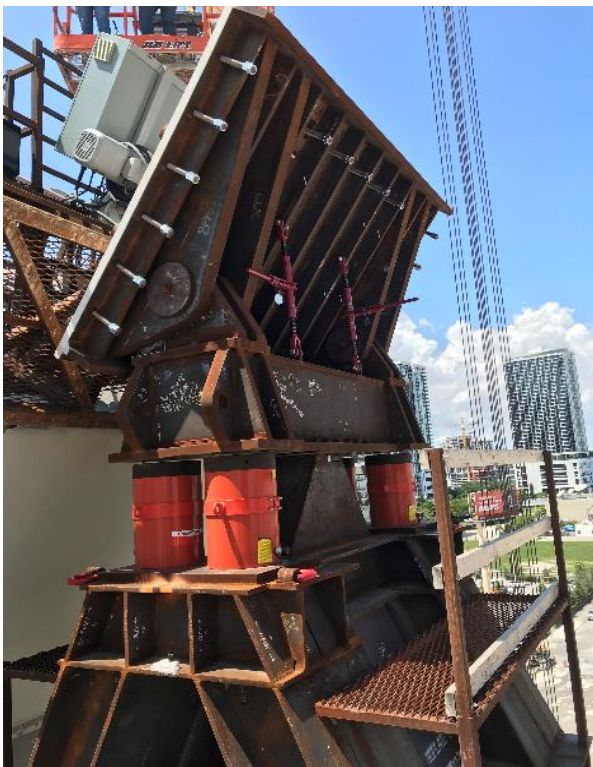
Figure 23: Temporary bearing at falsework tower. Hydraulic jacks below the bearing are used for fitup and vertical load adjustment. The bearing can rotate to match the profile of the arch.
