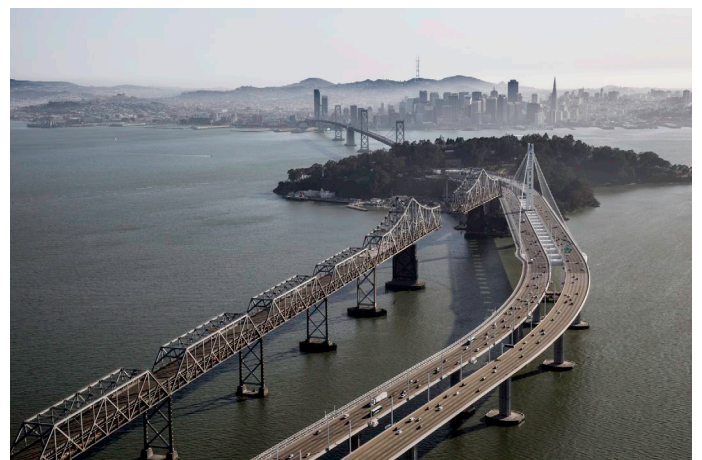
Aerial view of the SAS bridge under traffic while the original bridge began demolition
