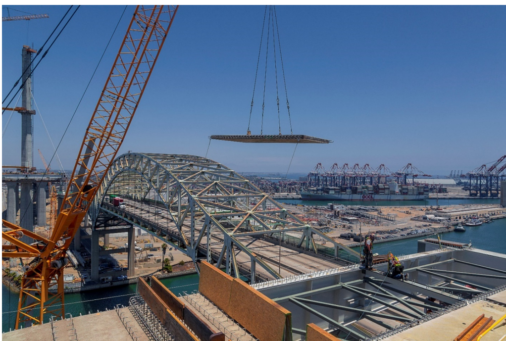
Figure 5: View of precast concrete panel being flown in for installation on the steel ladder-deck framing
