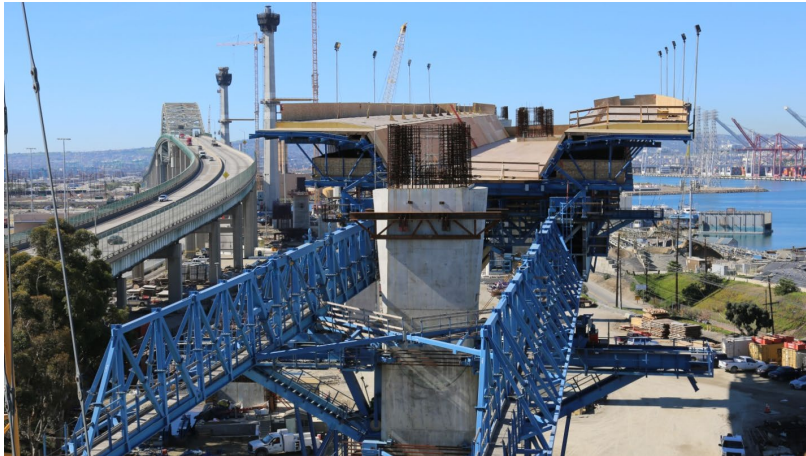
Figure 16: Underslung MSS ready for placement of reinforcement and prestressing. Photo courtesy of Marie Tagudena
