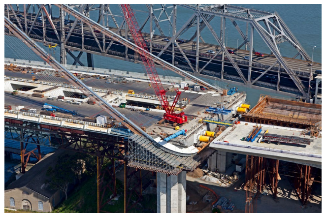
Close-up of looped cable west bent
