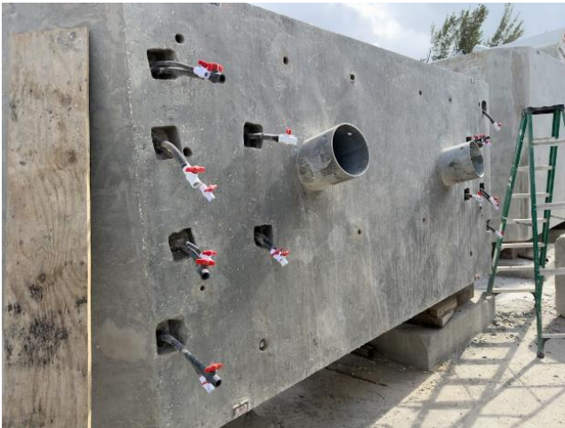
Figure 27: Intradados face of suspender segment. Guide pipes for suspender cables extend out of concrete. Grout tubes for vertical post-tensioning bars can be seen as well as the survey embeds along lower edge of joint.
