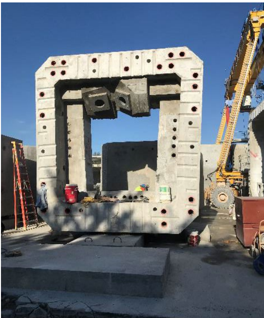
Figure 25: Suspender segment showing asymmetric cable anchorages. Note asymmetry in PT duct arrangement.
