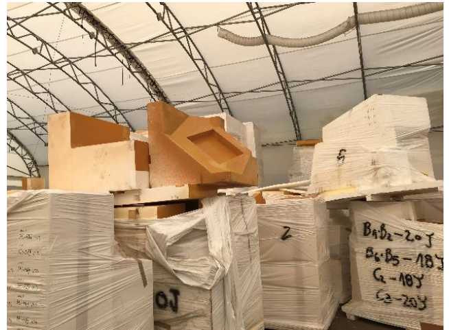
Figure 28: Foam void formers for suspender anchor blocks. Complex geometry is achieved by cutting foam blocks to shape using CNC router. This geometry is taken directly from the 3D CAD models.
