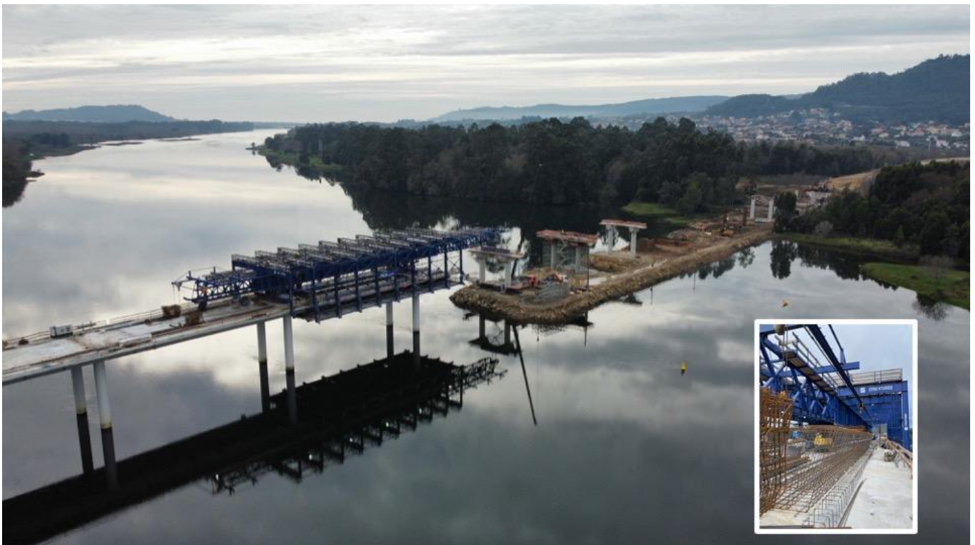
Figure 4: Overhead Movable Scaffolding System and detail of the transport of the pre-assembled reinforcement cage, Lima River, Portugal
