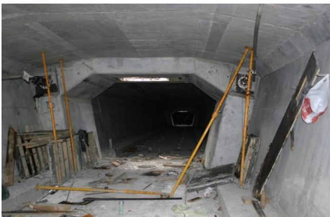
Figure 5: Opening in the diaphragm to allow the passage of the internal formwork
