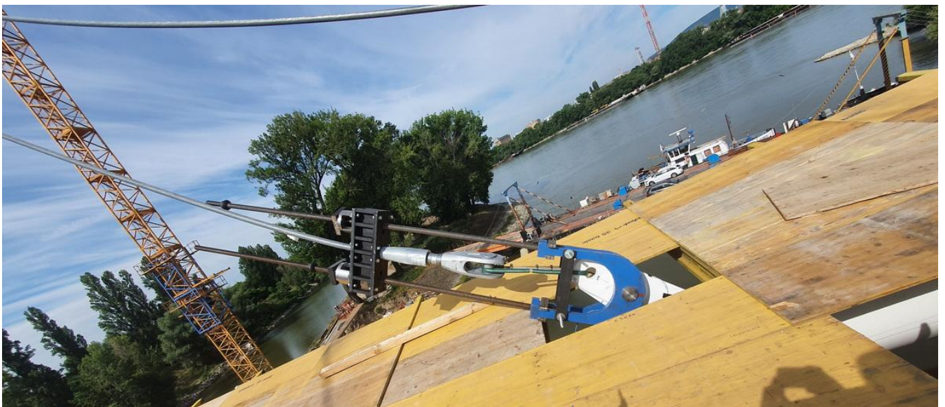
Figure 50: Cable tensioning device
